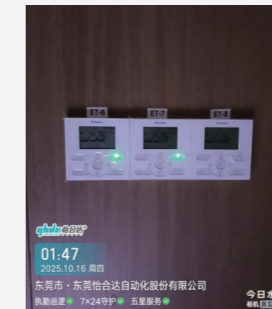
Air Conditioning Violation Inspection and Record-Keeping
