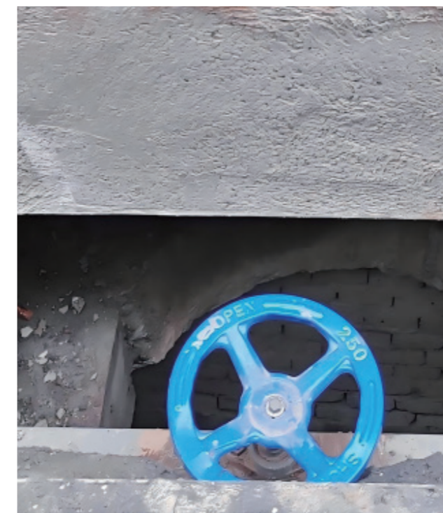
Rainwater Collection Network on the Factory Premises
