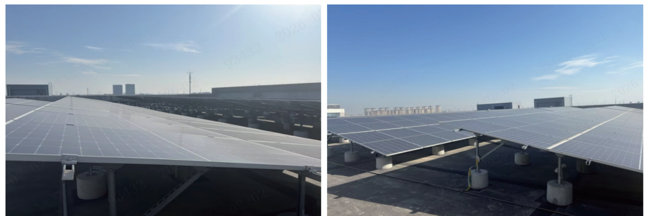
Suzhou Yiheda Production Base Photovoltaic Power Generation Project
