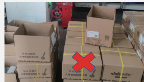
Goods Blocking Fire Safety Equipment
